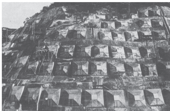
Figure 10. Example of the extensive use of permanent ground anchors in Hong Kong
